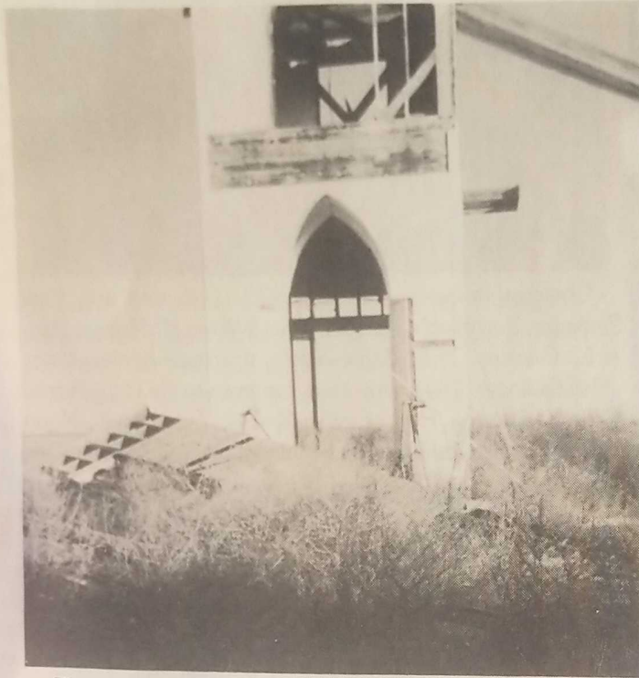
This picture was taken at the time when the church building was torn down, following the disbandment of the congregation. Shown is the entry and the base of the bell tower.
